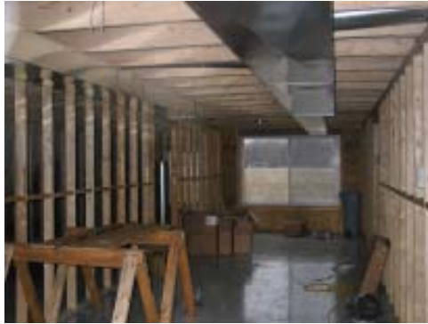
HVAC ducts, floor covering and a large window has been installed on the first floor of quonset hut #1.
