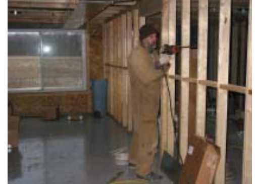
In quonset hut #1, Roger assists the electrician by drilling holes in the framing for the electrical wire.
